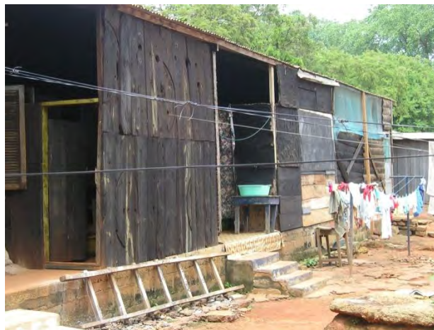
Figure 5: A timber house in a poor state
