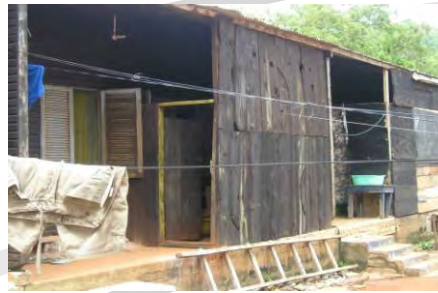
Timber houses in a poor state
