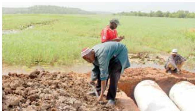
Farmers fixing a new culvert to address flooding at the Jahally rice field
