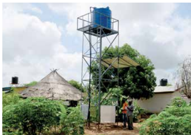
Water reticulation system at Kuntaur Health Centre
