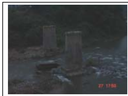
Photo 2. Only the foundations remain of the Hong Ha bridge over the Bo River that was swept away in the 1999 flood.
