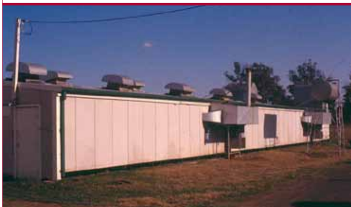
Oil or gas-fired hot air brooder units on side of shed for whole-house brooding: the entire brooding area is heated to the required temperature
