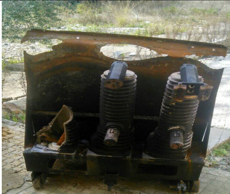
Figure 7: the damages of The spare access cell / 6.3 kV / within the Ain Al-Bayda hill transformer station
