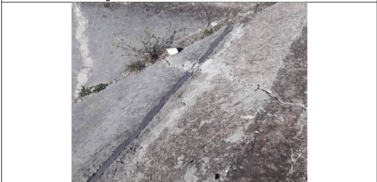
Figure 11: the damages of Fedrah water tank
