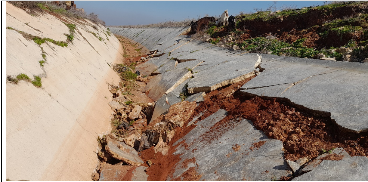
Figure 3: Earthquake caused damages (Downstream location of the damaged part of the PS)
