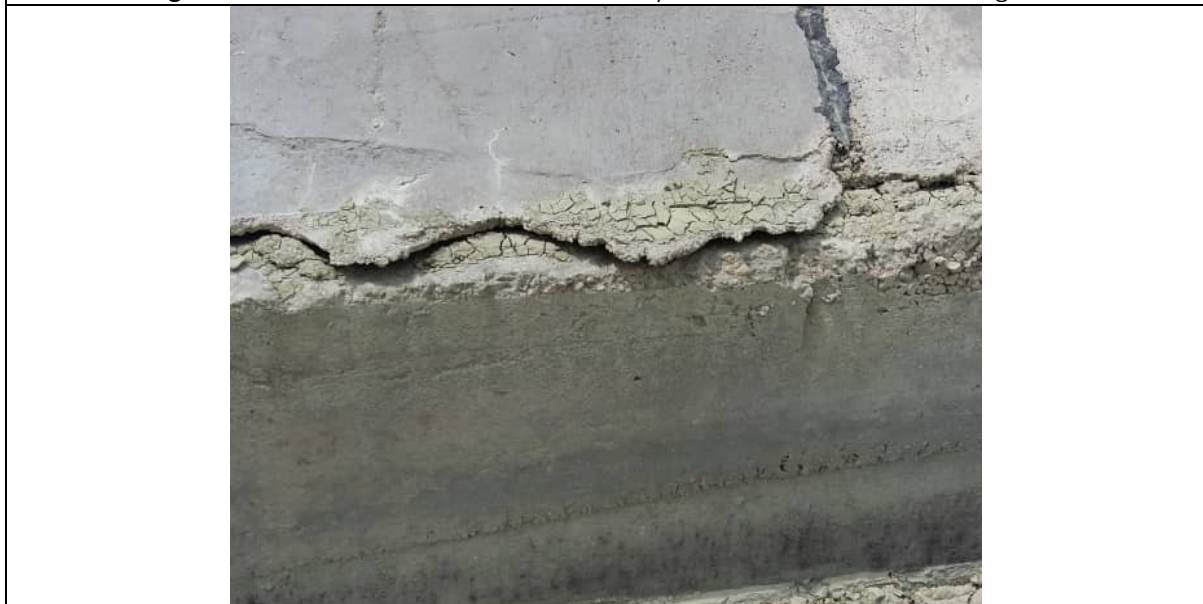
Figure 13: the damages of Salem Kharayib Small rainwater harvesting dam
