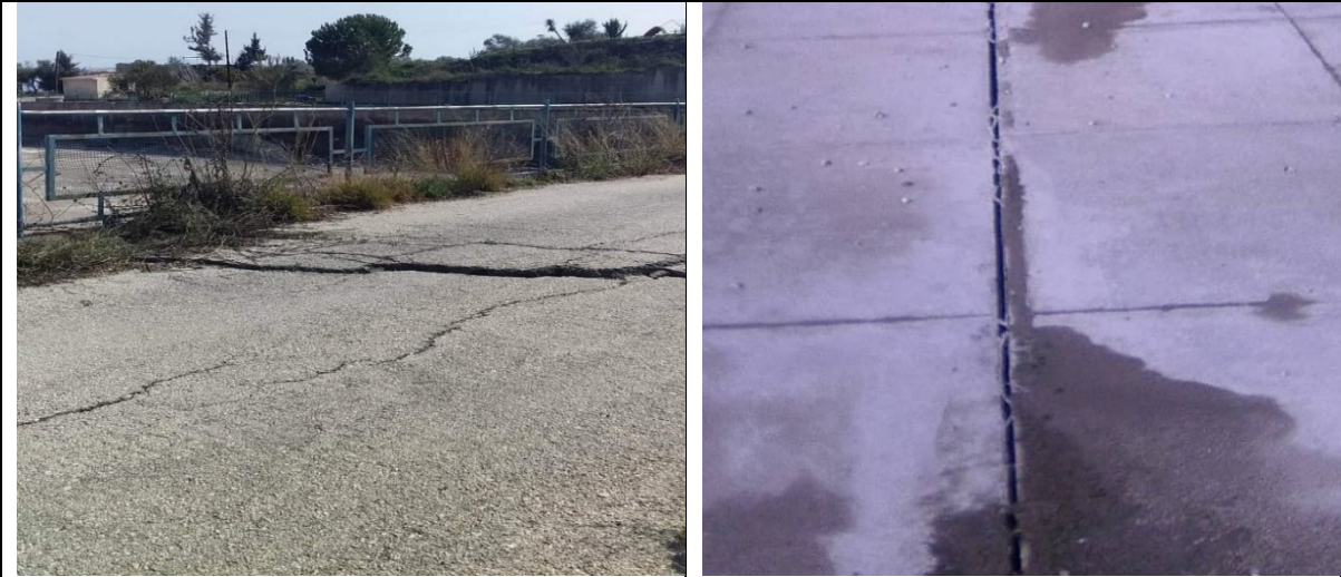
Figure 6: the damages of Qasmin water tank by earthquake
