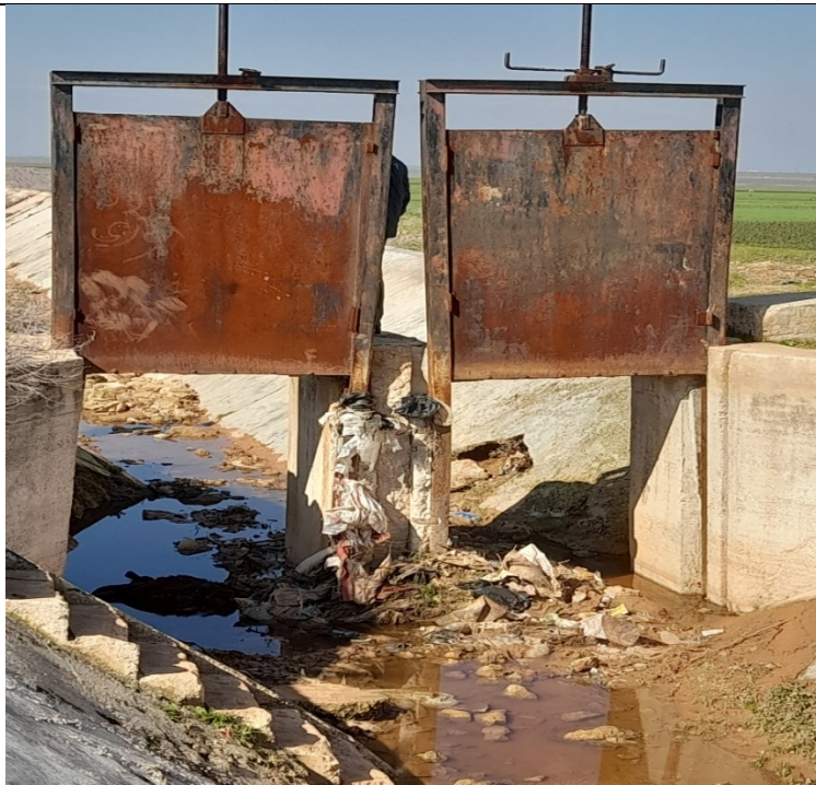
Figure 4: Earthquake caused damages of irrigation flow regulator on primary canal, PS
