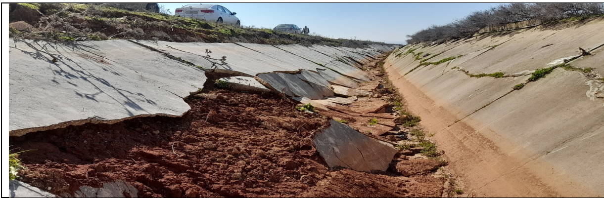
Figure 1: Earthquake caused damages (Upstream location of the damaged part of the PS)
