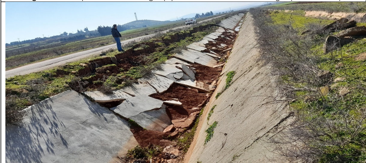
Figure 2: Earthquake caused damages (Location on the middle of the damaged part of the PS)
