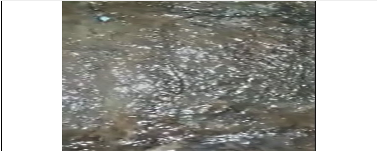
Figure 9: the damages of seventh inverted siphon (this photo inside the siphon)
