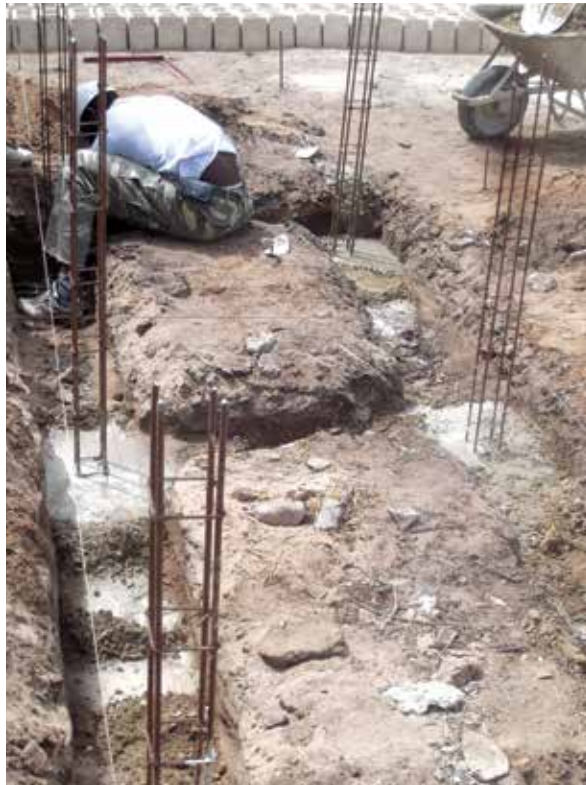
5 - Iron bars are positioned in the trench. The foundation is then cast
