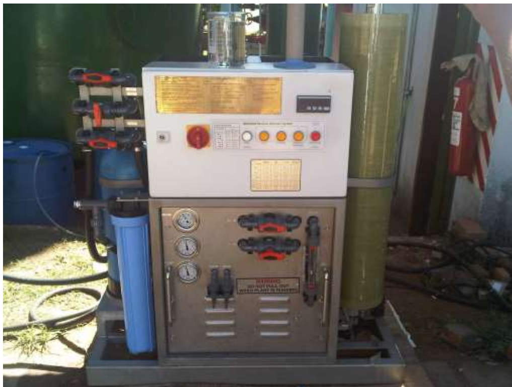
Figure 2: Modular equipment PT-RO
