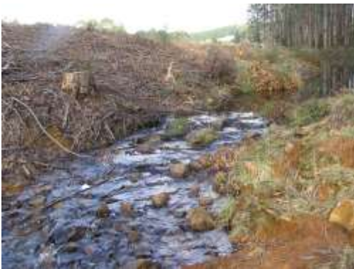
Figure 3: Harvesting up to stream edge without disturbing soil, using a 10 m machinery exclusion strip
