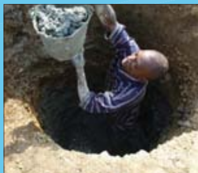
FIGURE 3. Open well development and lining with concrete rings – SPFS in Sierra Leone
