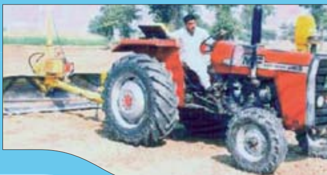
FIGURE 44. Precision field leveling in the OFWM Programme in Pakistan – Government of Punjab
