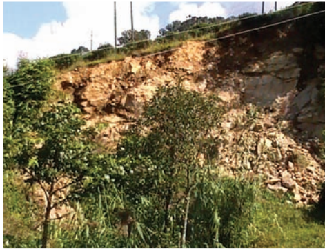
Landslide on Monteviot tea estate (close view)
