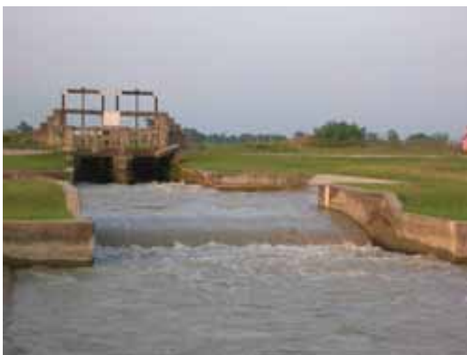
Plate 28 Head of secondary canal equipped with a measurement device (gauge) of very low accuracy (Nepal).
