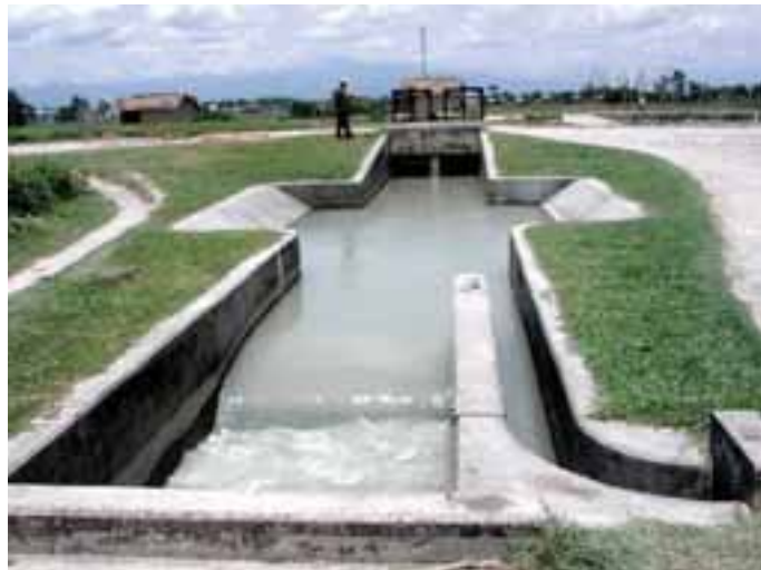
Plate 18 Dysfunctional proportional divider (Nepal) with different downstream conditions: free-flow (main branch left) and submerged (small branch right). The capacity of the structure with respect to proportional division is at stake.
