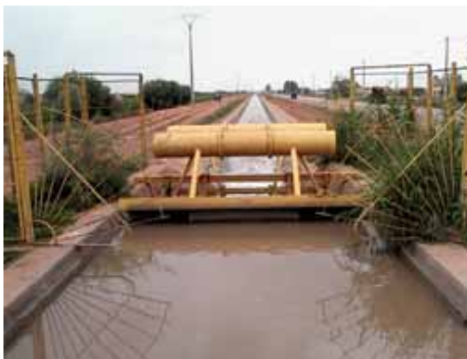
Plate 6 A self-acting upstream control gate (AMIL gate).
