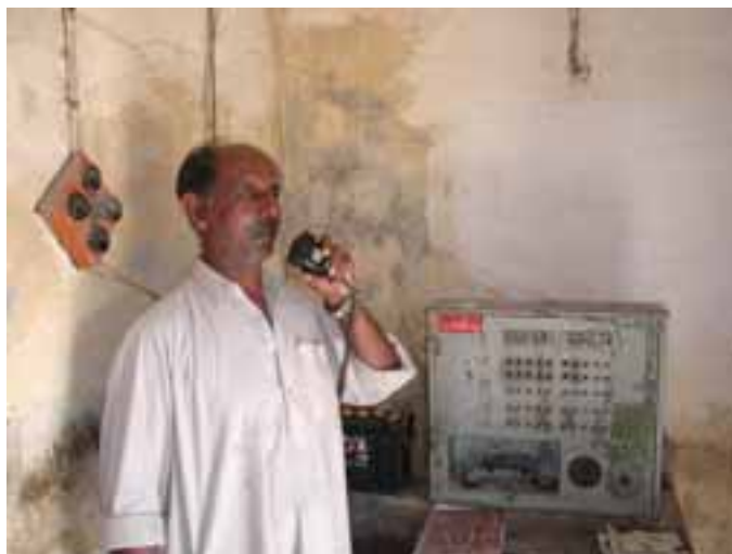
Plate 21 An operator using an old communications system in the Nara Canal, Sindh, Pakistan.
