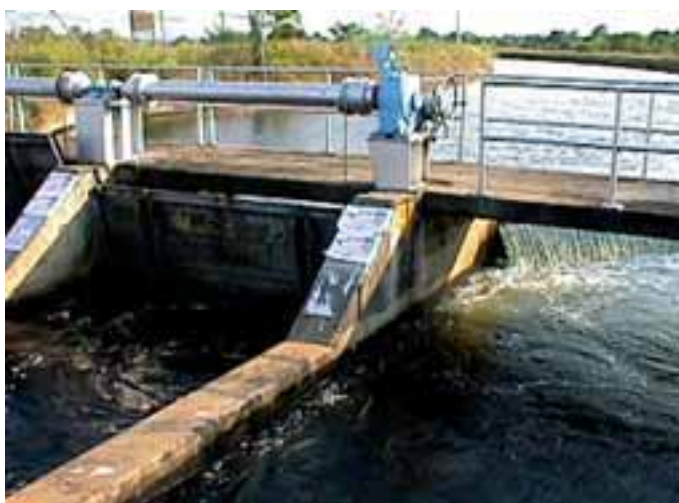
Plate 9 Cross-regulator equipped with central radial gates and side weirs, Mahaweli B, Sri Lanka.
