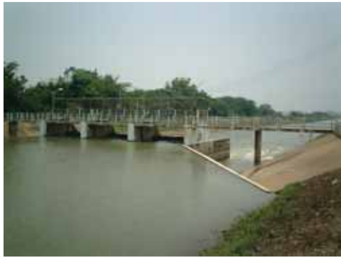
Plate 23 Mixed cross-regulator with undershot middle gates and side weirs, Thailand. The functioning of the regulator is not appropriate – water should spill over the crest.
