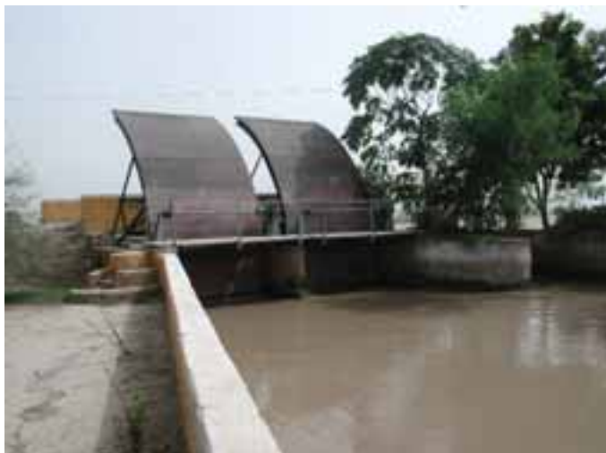
Plate 11 Dysfunctional cross-regulator along a main canal in Sindh, Pakistan – radial gates are blocked fully open as they cannot be closed because of design problems.
