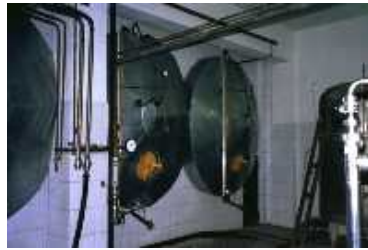
Beer cooling tanks
