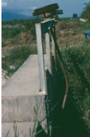
Photo 1 Dominican Republic: A tampered gated check structure
