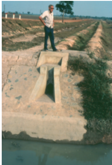
Photo 2 Canals designed for operation at full supply cannot deliver water to the lower level because of a lack of check structures
