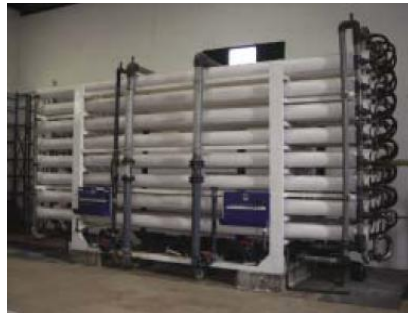
Figure 1. A 2 500m 3 /day Reverse Osmosis Plant Treating Brackish Groundwater in Spain (by membrane technology)
